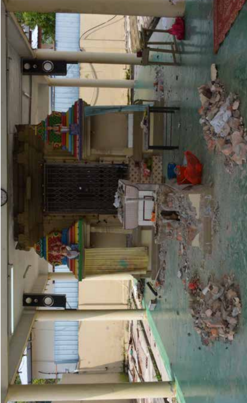
Figure 6.2. Demolition in progress, the Sri Maha Mariamman Temple, Mengkitbol, 2017. © Ravinran Kumaran, used with permission
