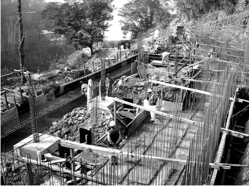
Figure 1.3. Reconstruction in Mountainous Areas. Most of the reconstruction in this project was in mountainous areas on small plots of land, such as this AJ&K location. Here, construction work underway was being inspected. Government Girls' Middle School Kahna Mohri. 2007. © Zahid Ur Rahman.
