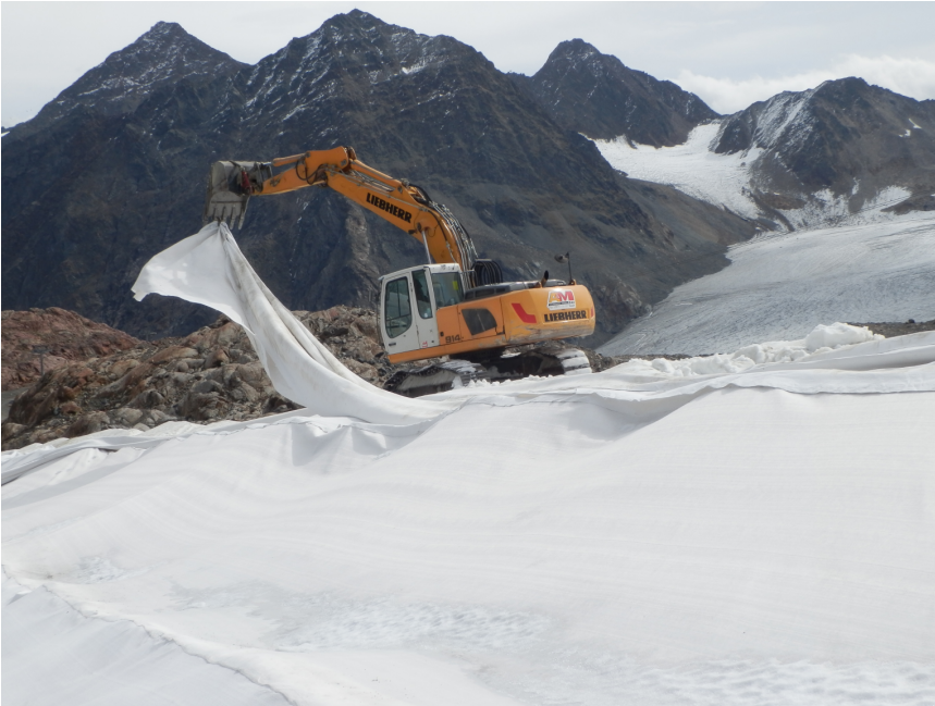
Figure 9.2. A worker uses a digger for removing some textiles in late summer 2015. © Herta Nöbauer.
